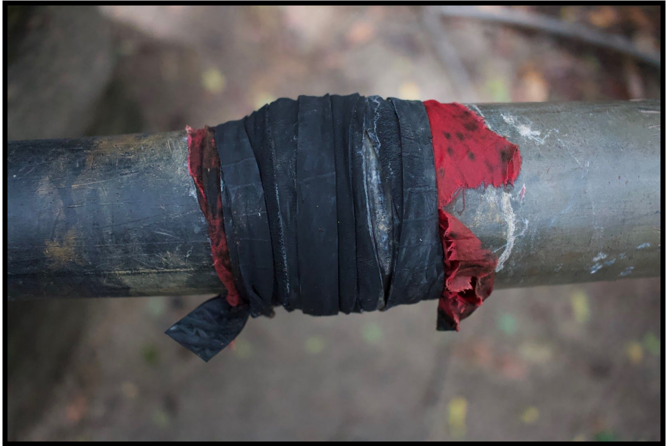
Figure 3.2.1: Common repair to the government system (James Trebesch, January 2018)
