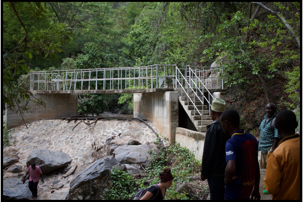
Figure 3.2.2: A portion of the aqueduct used for agriculture and the piping for village water (James Trebesch, January 2018)
