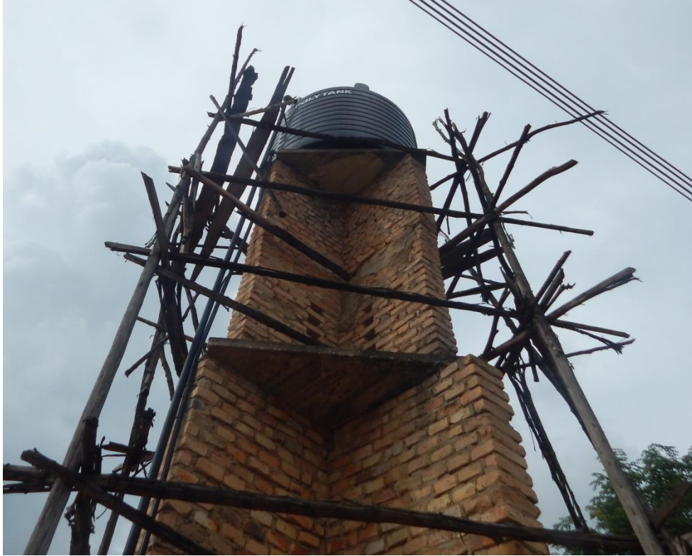
Figure 4: 5,000 L tank on 8 m water tower
