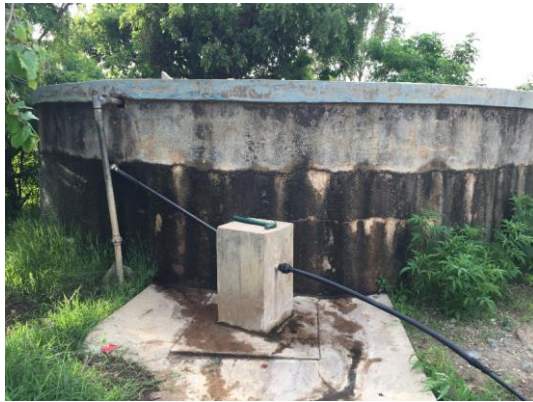
Figure 4: 32kL Concrete Tank with Large Crack
