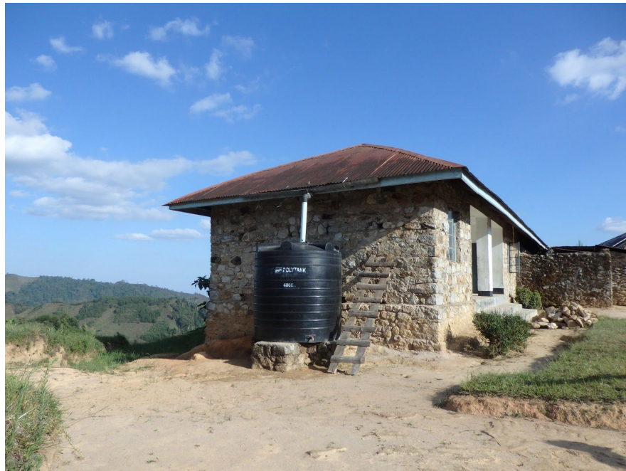
Figure 3.7: The 4,000 L water tank on the side of the dispensary was poorly designed for rain catchment. The dispensary is located at 8.201781 S, 36.045606 E.
