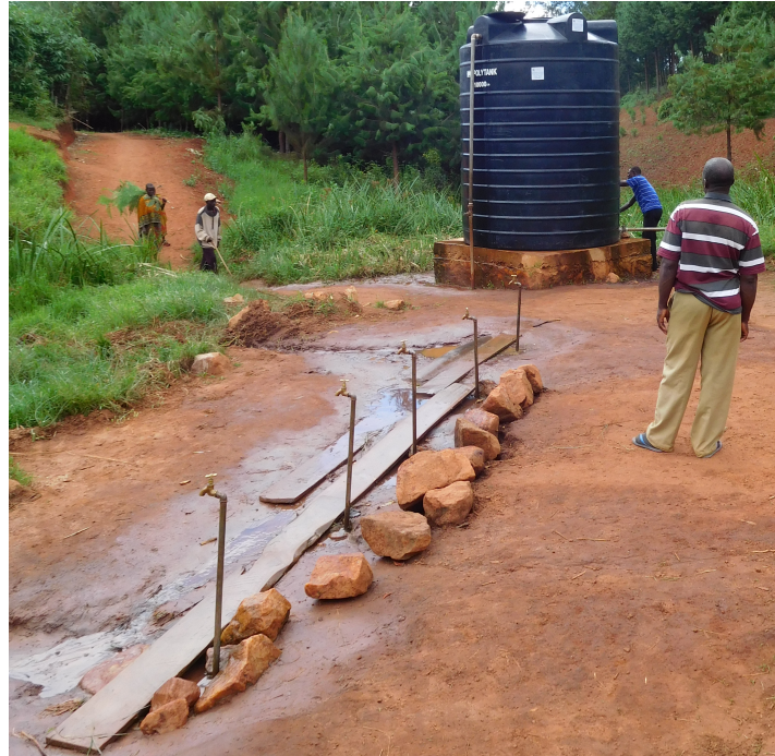
Figure 4 - Current Tank and 5 Spigots installed in University of Minnesota Student Designs in 2014.
