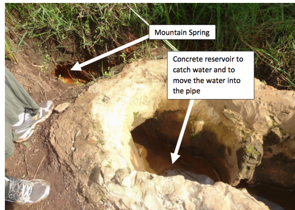
Figures 15: concrete basin used to collect water exiting the mountain source
