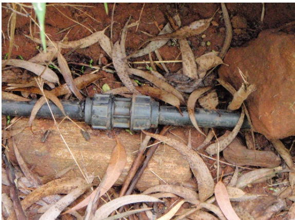
Figures 14: photograph of exposed pipe connection on Sajeni line
