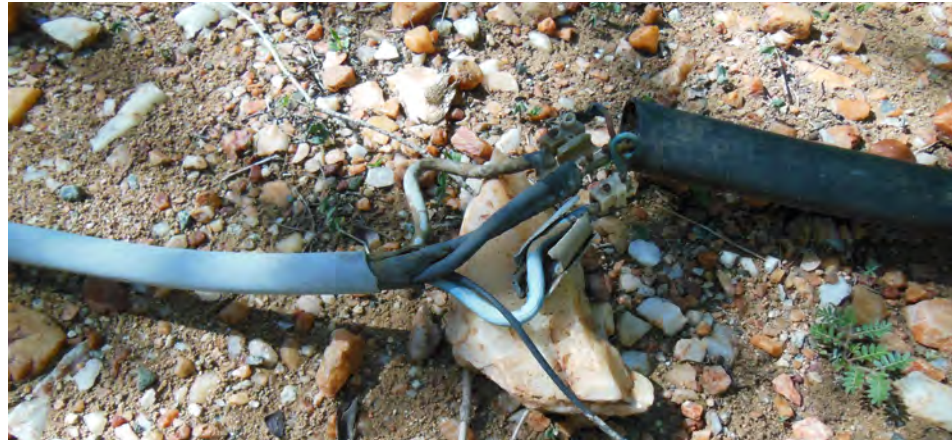
Figure 9: Exposed wire splice. Located on the east side of the school grounds.
