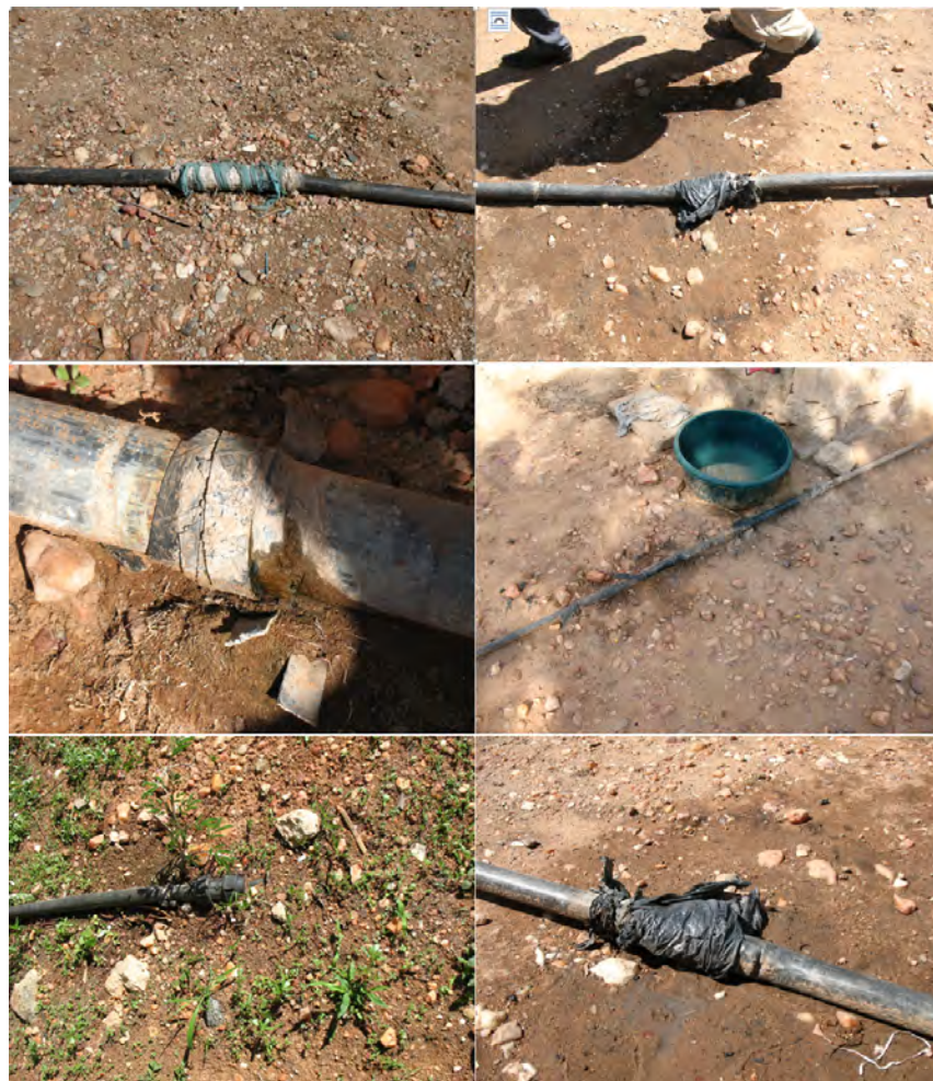
Figure 4: Disrepair at various points in the current pipe system. Bottom left: HDPE system intake pipe; bottom right: GS system intake pipe; middle left: GS system intake pipe; middle right: GS system pipe near staff buildings; top left: HDPE pipe originally use.
