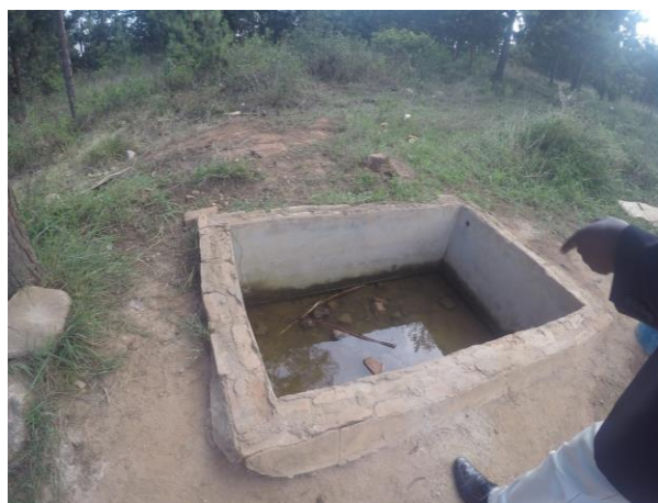
Figure 2.3.2 New Tank Location in Ibwange. The piping is currently connected to a collection ditch. The placement of the tank would be near this location which is on the south side of the school.
