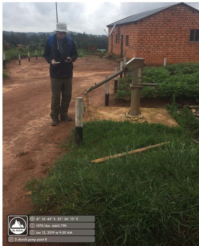
Figure 5: Hand pump adjacent to Lutheran church. Well depth is 24.4 m and the original water level was 10.7 m. Ran dry in 2016.
