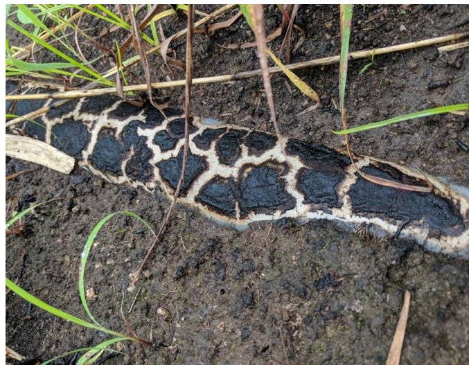
Figure 9: Burnt pipe observed on gravity main running through farmland in Nyamagola A.
